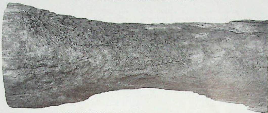
UNTREATED PINE PILE—BOCA GRANDE, FLORIDA Work of Linnoria . The pile was two years in service.
