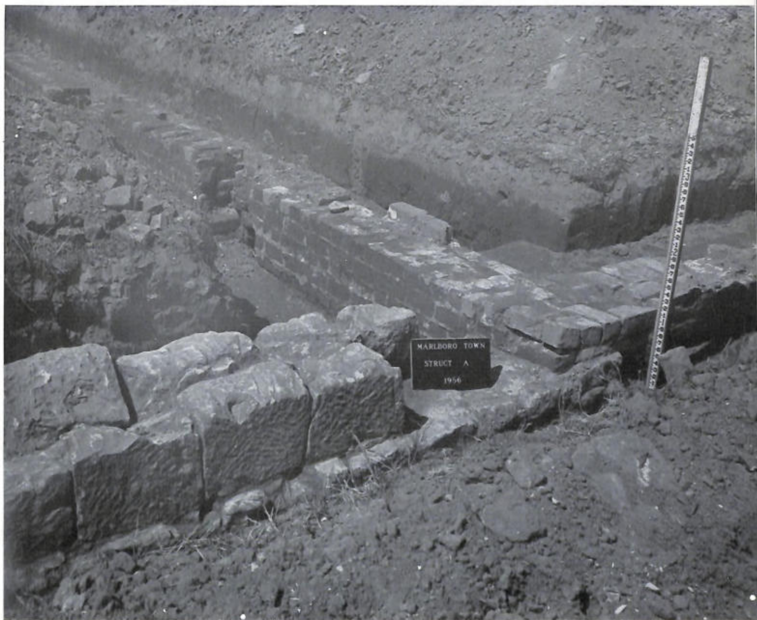
Figure 24.—JUNCTION OF STONE WALL A, running from creek side to this point, with brick Wall A-I at top left, Wall A-II at right.
