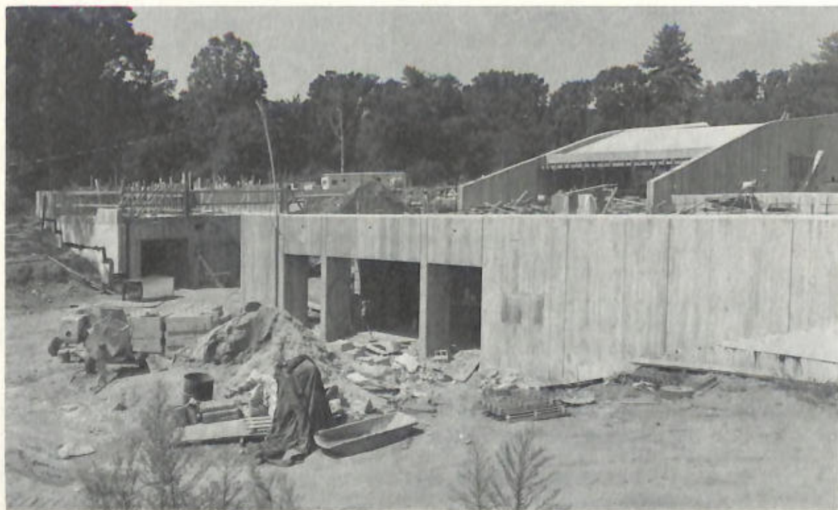
21. This 1975 photograph shows the entrance of the Lion-Tiger Exhibit during construction. Nine months later, the building and viewing areas were completed and opened to the public.
