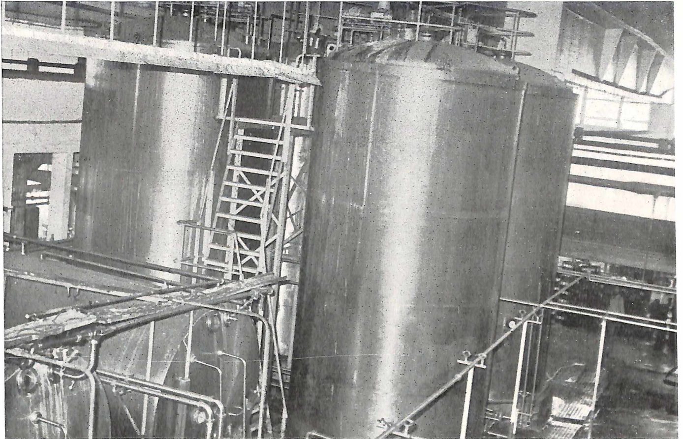
Milk storage tank inside the Mother Dairy at Dankuni
